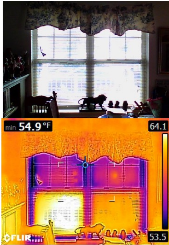
Thermal bridge and air leakage around windows
