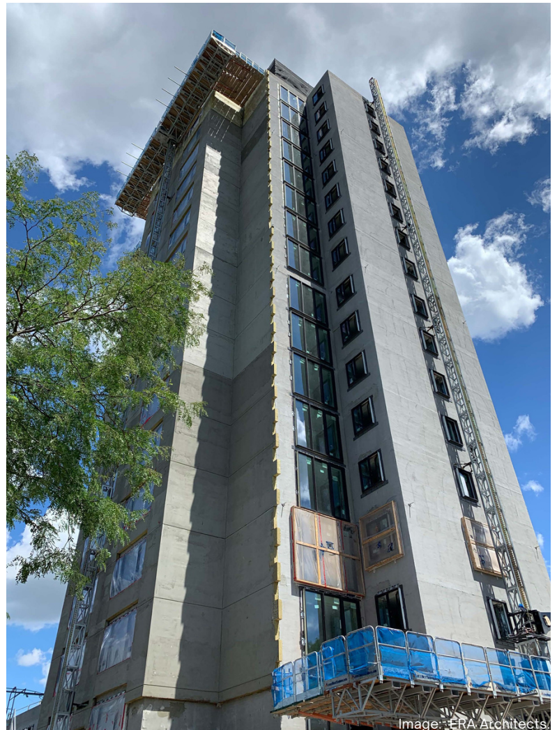
Construction on the exterior envelope including window and "Juliette" balcony installation (right). Interior view after construction (left).
