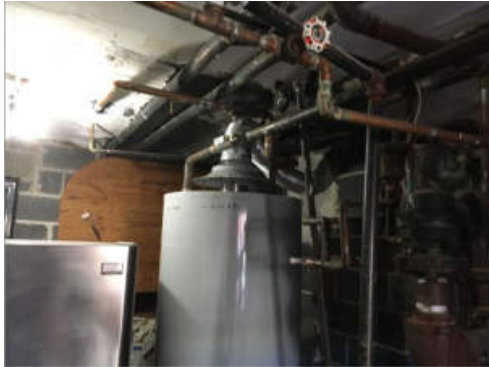
Existing Gas Water Heating
