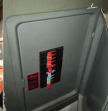
Existing 40 Amp Panel in Unit
