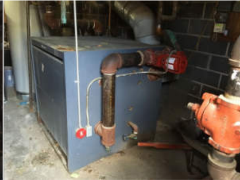
Existing Centralized Gas Boiler for Heating
