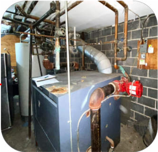
Existing boiler and gas HW heater
