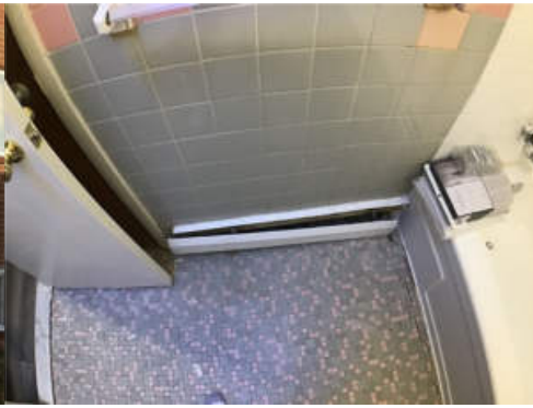
Existing Hydronic Baseboard Heating
